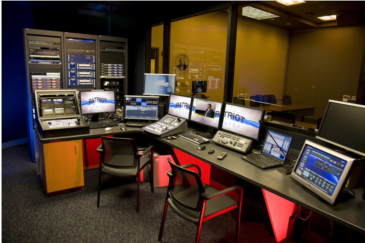
The Auditorium Control Room of new Patriot Center – Lockheed Martin Space Systems Company, Newtown, PA
